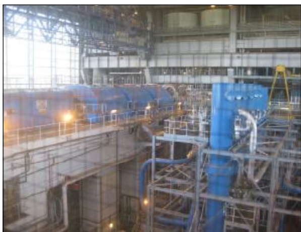
One of the Turbine Generators on its Concrete Foundation at Ironbridge B.
