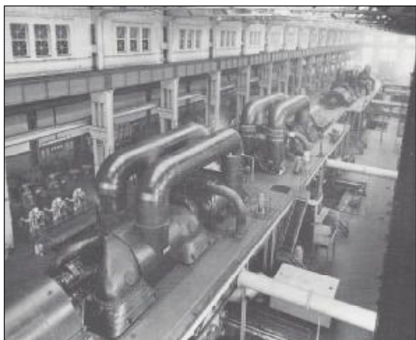
Ironbridge A Turbine Hall with 4 Turbines installed.
